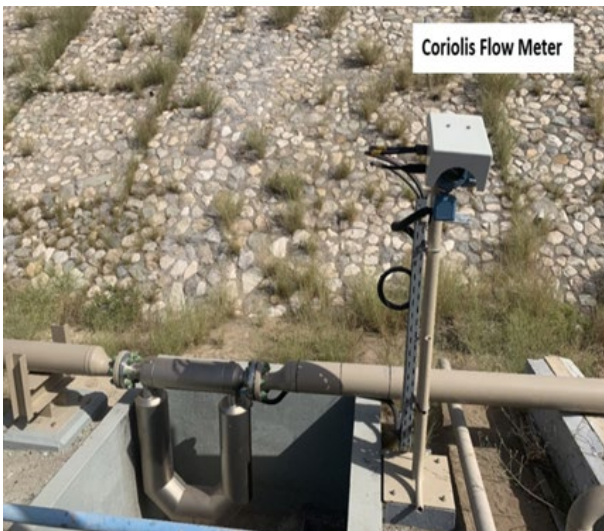
Figure 3. Sensor locations on a 6'' pipeline
