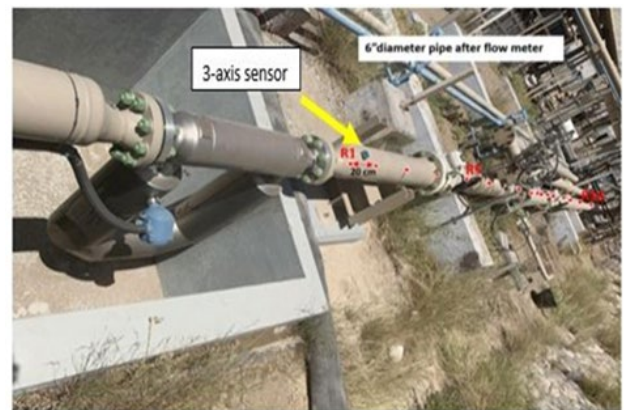
Figure 2. Sensor locations on a 6" pipeline
