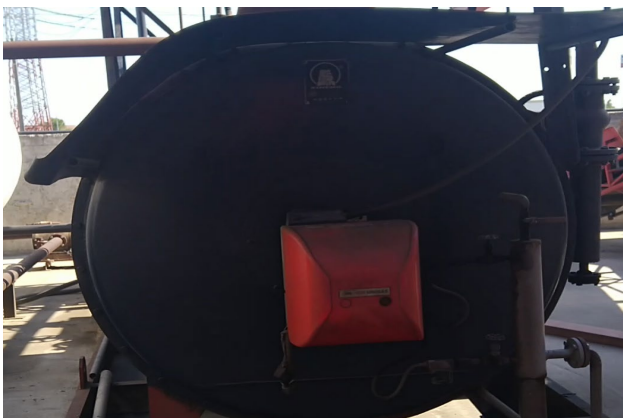
Figure 6. Thermal oil boiler and burner assembly
