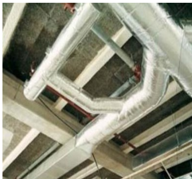
Figure 9. Exhaust and hot air ductwork insulated with mineral wool blankets
