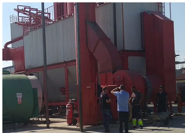
Figure 10. Sound-absorbing barrier wall encompassing major mechanical noise sources
