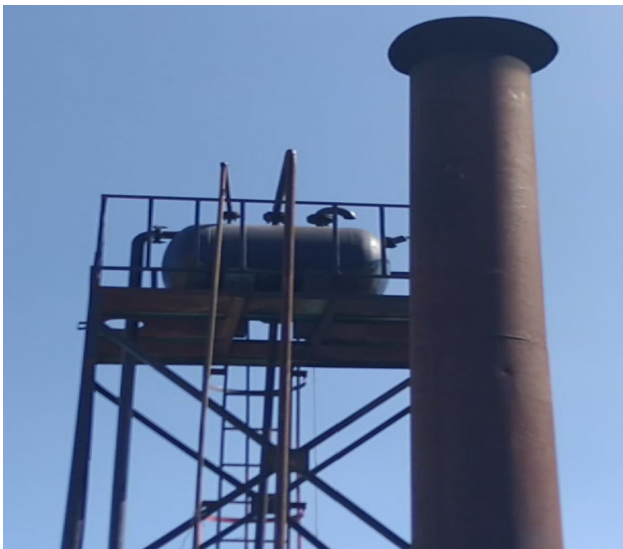
Figure 5. Exhaust stack for combustion gases from the asphalt plant
